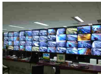
苏州北环隧道监控 Suzhou Tunnel Monitoring System
