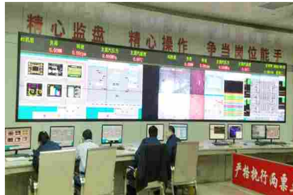
常州电厂 Changzhou Power Plant
